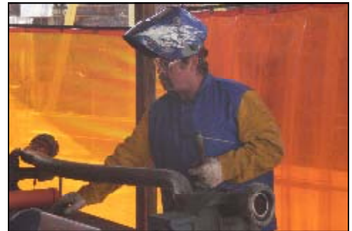
Some of the larger piping on 2926 does not need replacing, but must be repaired. Here Local 412 member Randy "Big Dawg" Aderhold begins work on a very crooked pipe.
